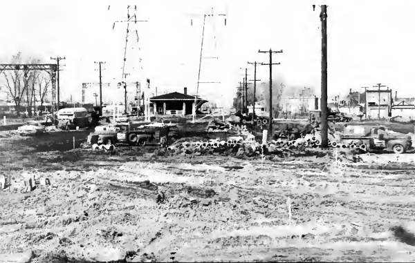
By March 1964, the Park'n'Ride lot contractor had completed rough grading and was installing the drainage system. Early spring snow then made paving work impossible for several weeks.
